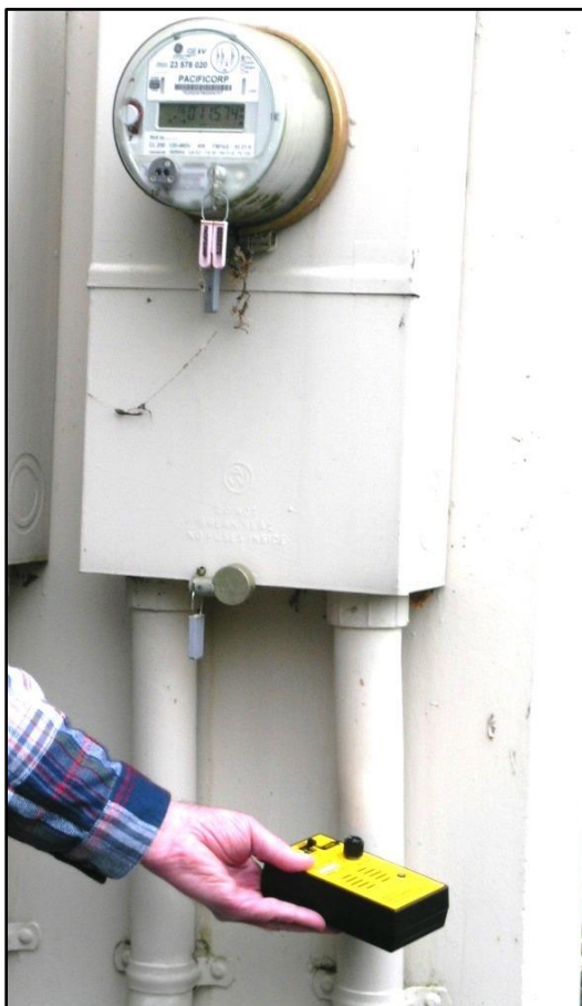
(FIG. 2) PROBING THE METER
